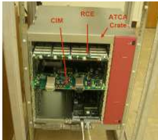
Figure 2.56: ATCA Crate with RCE and CIM.
